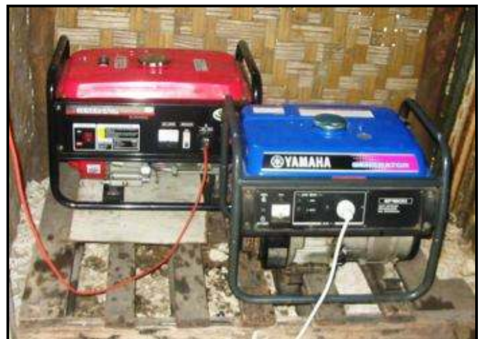
Generator financed by Micro loan – Atchin Island
