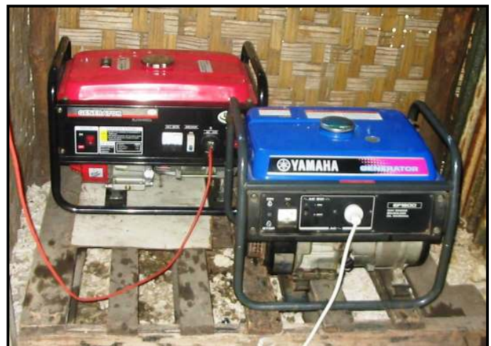
Generator financed by Micro loan – Atchin Island
